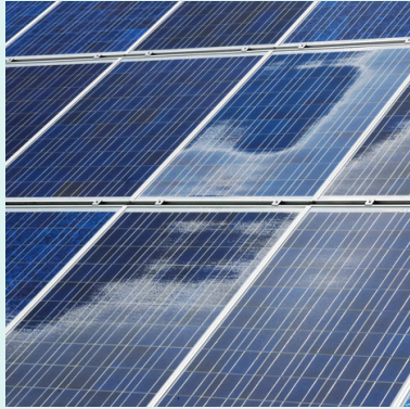
PHOTOVOLTAIC SYSTEM FOR EVERY FLAT
